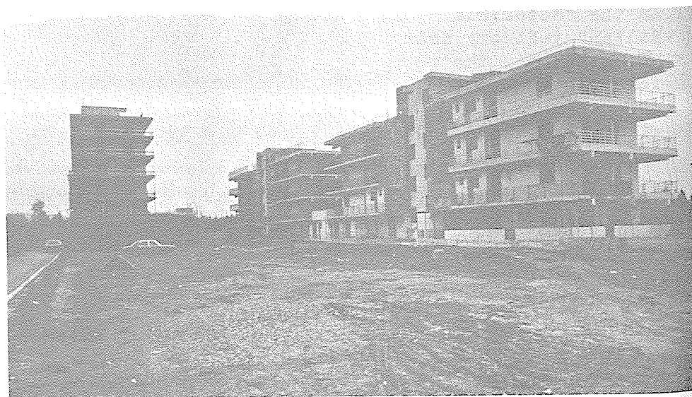
14: This building with holiday flats on the Bay of Loutraki was severely damaged but could still be lived in.
