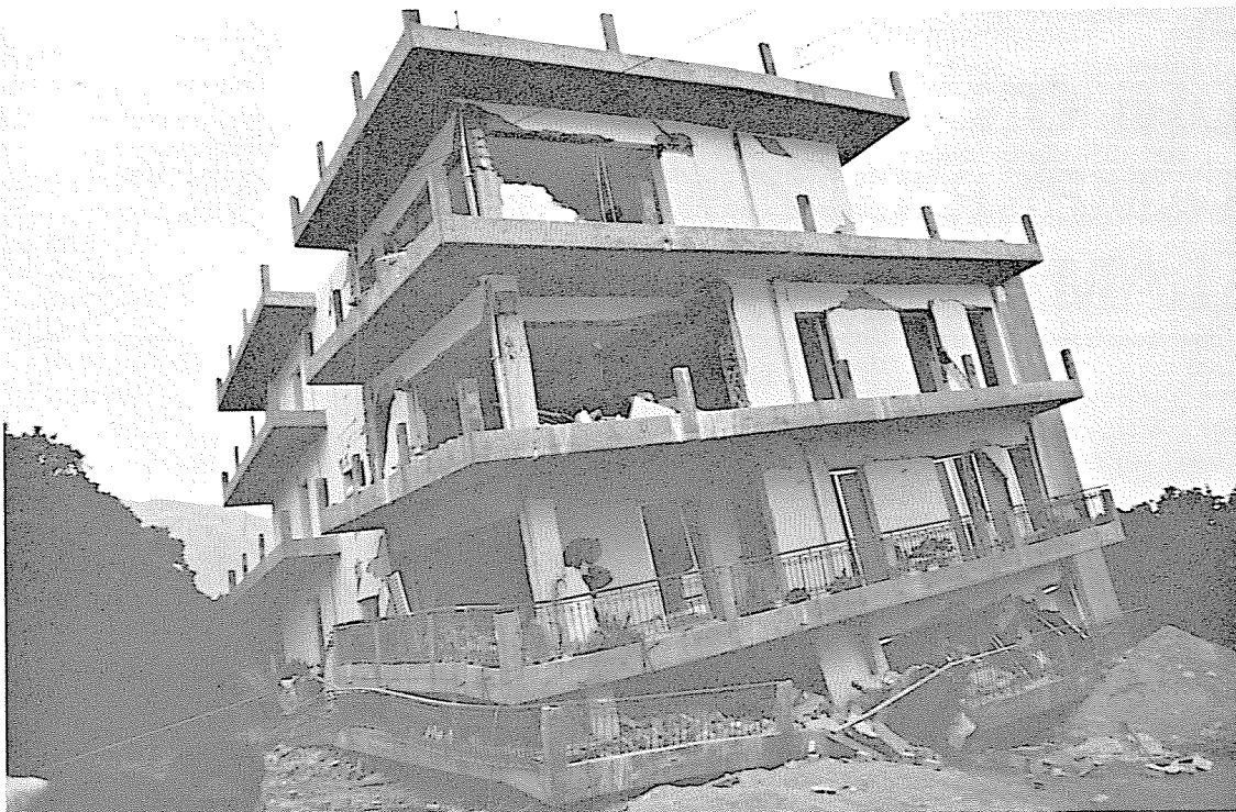
Figure 2. Partial collapse of a five-story reinforced concrete apartment building. The partitions are brick walls. The building was brand new.
