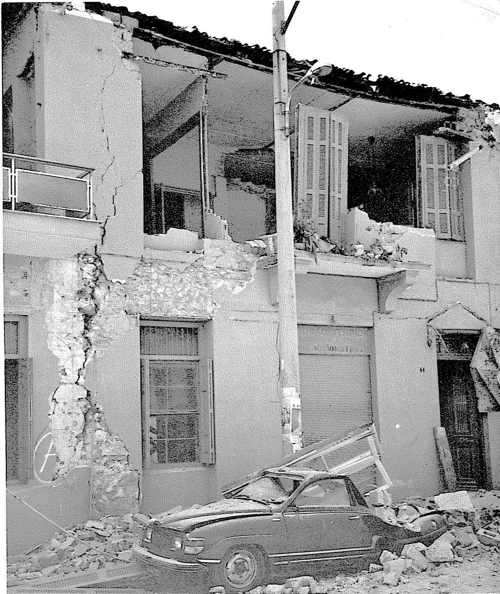
Figure 7. Many cars were damaged by fallen facades.
