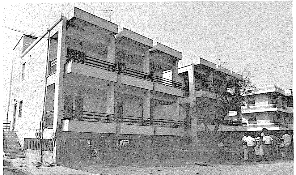
Figure 4. Two almost similar buildings behaved quite differently. The one at the left experienced extensive damage in the "short columns" of the basement, coming to rest as though torsion behavior had been prominent.
