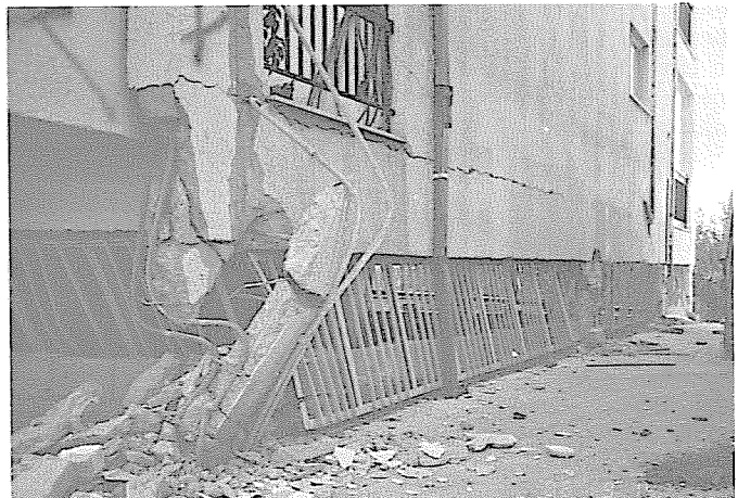
Figure 9. The front, right-hand corner column of the damaged building on the left in Fig. 4.
