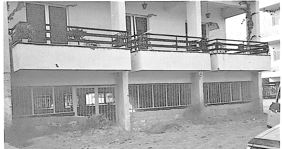
Figure 5. The building on the right hand side of the previous figure survived the earthquake with very small cracks.
