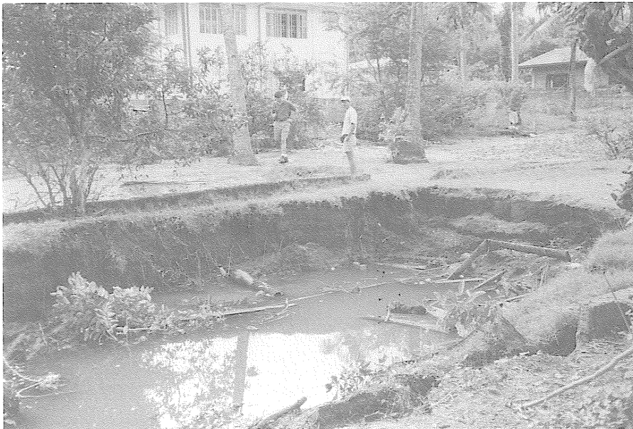
Figure 5—Large collapse near airport and beach area formed in dirt road by venting of sand into low-lying area at right side of photograph. Road constructed on loose fill placed on sand deposits. Throat of sand boil is in center of photo, at rear. Note shallow water table and large volume of sand expelled towards top of photo.
