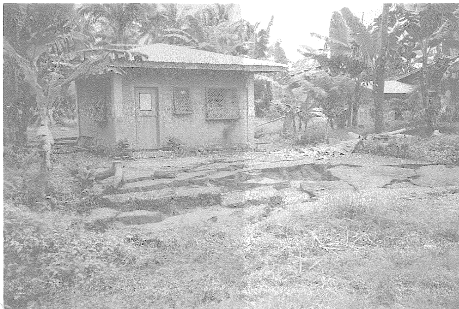
Figure 4—Liquefaction and lateral spreading cracks developed in a low-lying fluvial floodplain. Site is located within 1 km of the surface rupture. Note absence of damage to small concrete frame and hollow block structure.
