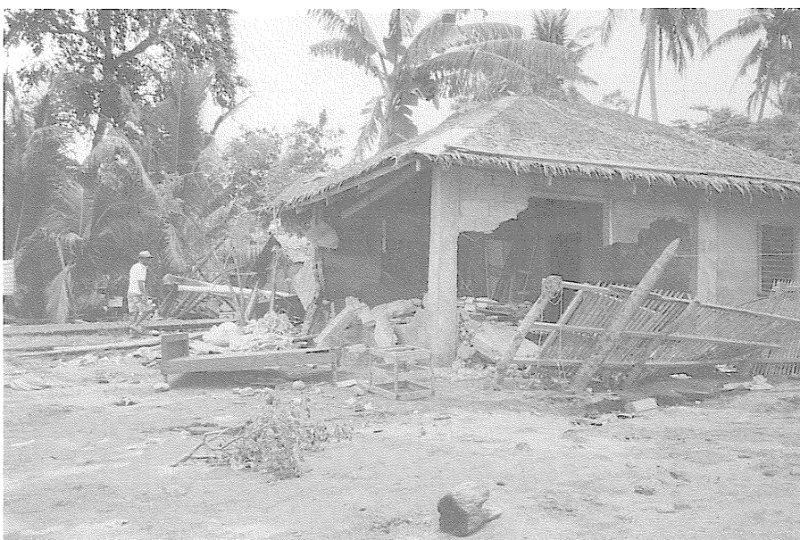
Figure 3—Severely damaged residence in the coastal town of Wawa. The tsunami was estimated to have attained a vertical runup of 2.5 m and a horizontal runup of 200 m in this area. The wave apparently exited back to the sea as indicated by the direction of compressed grass and bushes.
