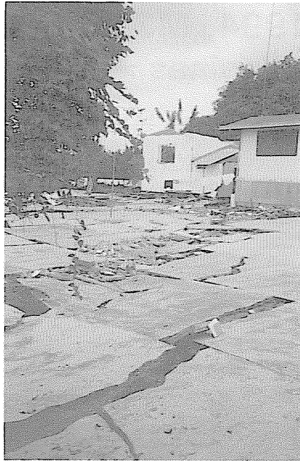
Figure 2—Trace of fault rupture as it passed through a residential lot, shattering concrete slab and displacing adjacent buildings. Fault movement in this area was slightly more than 2 m horizontal and 0.3 m vertical. Damage to these buildings appeared to be largely related to ground displacement rather than a result of strong shaking.
