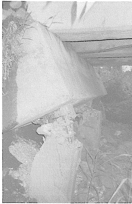
Figure 7—A simply supported, reinforced concrete deck and girder bridge that was badly damaged as shown by the severely rotated seat-type abutment with broken piles. Area is within 2 km of the fault in an upland terrace area. Damage to nearby concrete frame and hollow block structures indicates that this area experienced significant strong ground shaking, as well as extensive liquefaction and lateral spreading.
