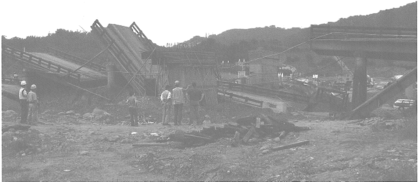
Figure 14 - The fault ruptured beneath the I-Jiang Bridge, about 30 km NNW of the epicenter. (Photo: Moehle)
