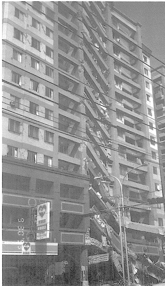
Figure 12 - View of a partially collapsed 15-story building (less than 50 m high). Reinforced concrete with infill brick partitions. Beam column joint failure at facade.
