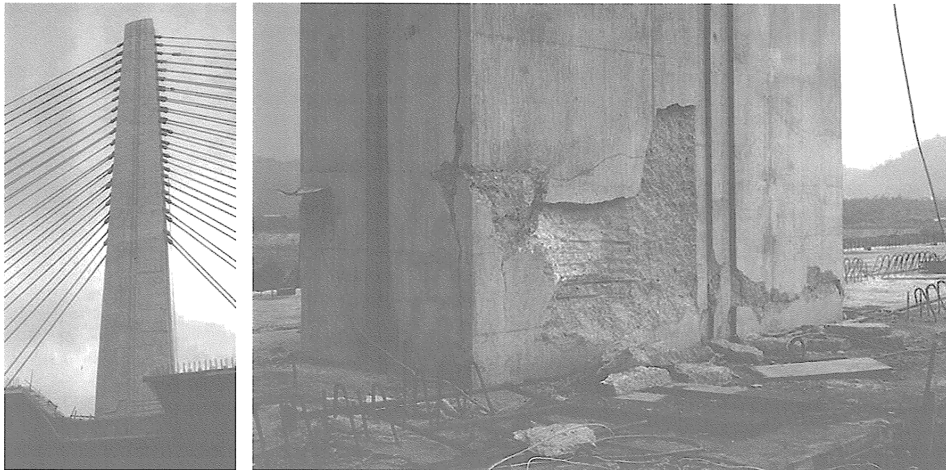
Figure 15 - The Jyi-Luh cable-stayed bridge, about 10 km SW of the epicenter, was under construction and sustained significant damage. (Photo: Moehle)
