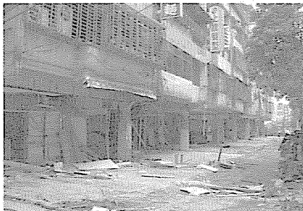
Damage to residential building in Taiwan. Check EERI's Housing Encyclopedia for a complete description of this construction type.
