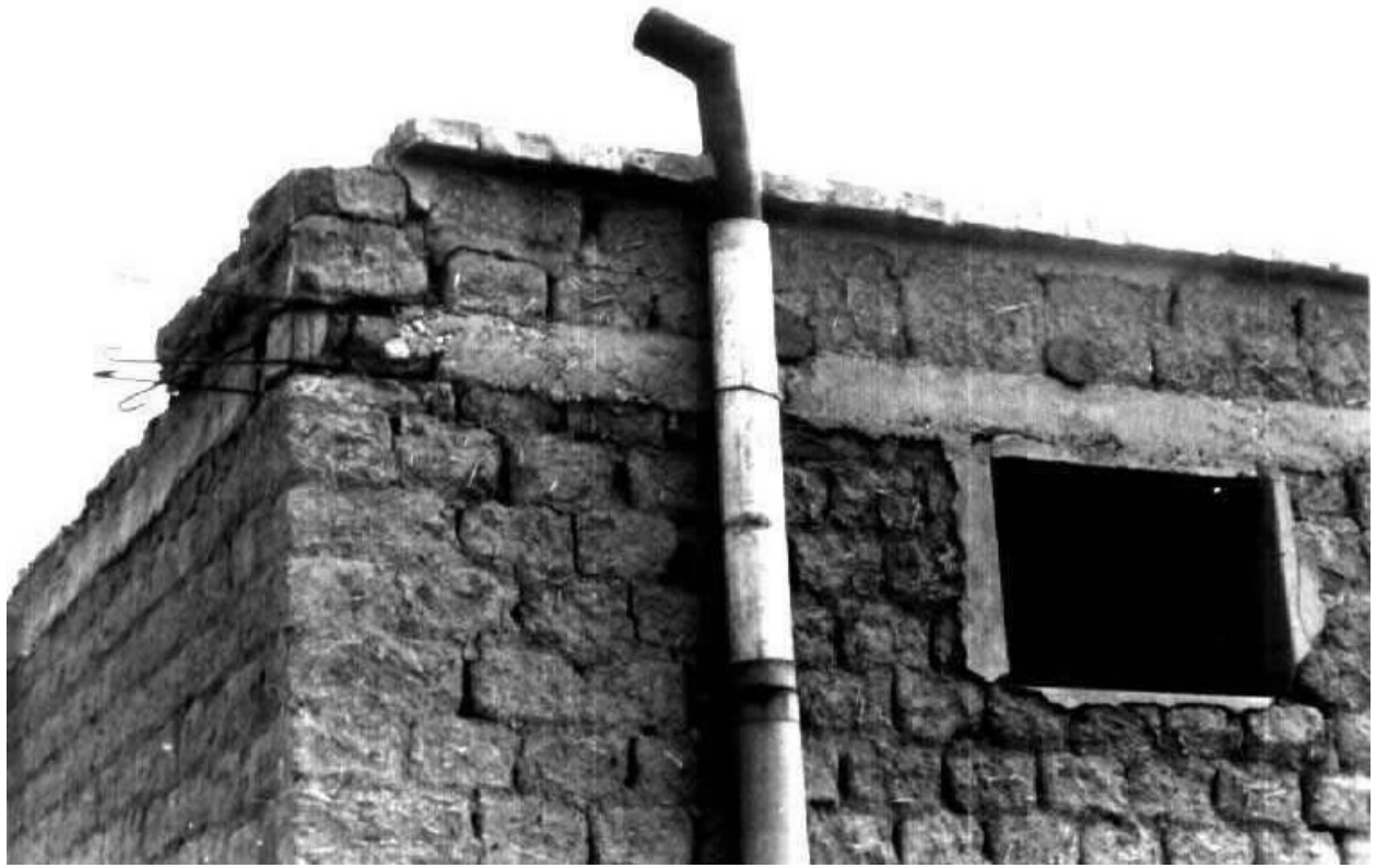
FIGURE 6B: A Photograph Illustrating Typical Earthquake Damage
