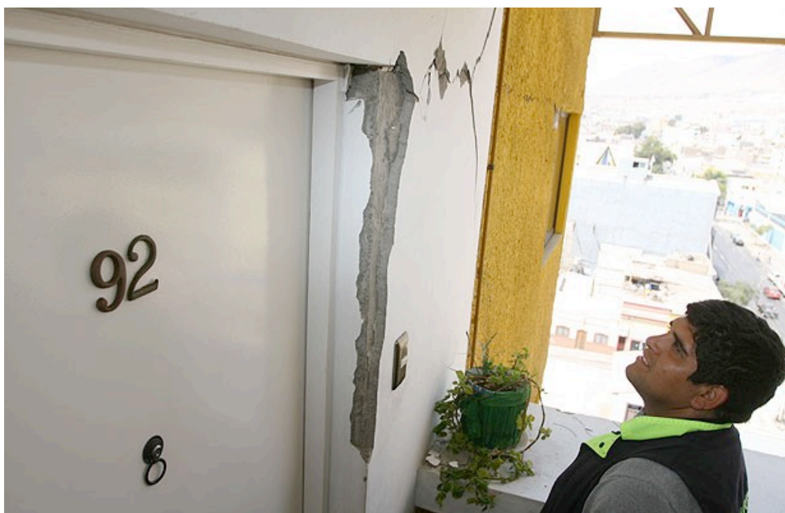
Figure 8. Structural damage in a building (Source: www.emol.com )
