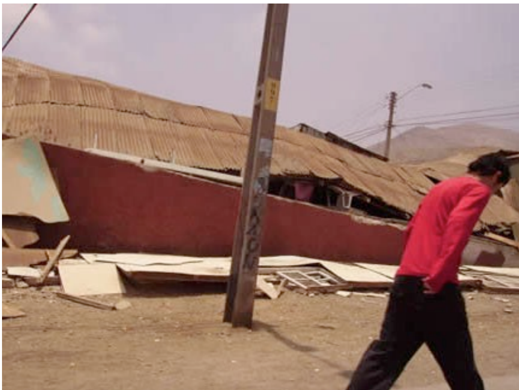
Figure 7. Wall collapse (Source: www.emol.com )
