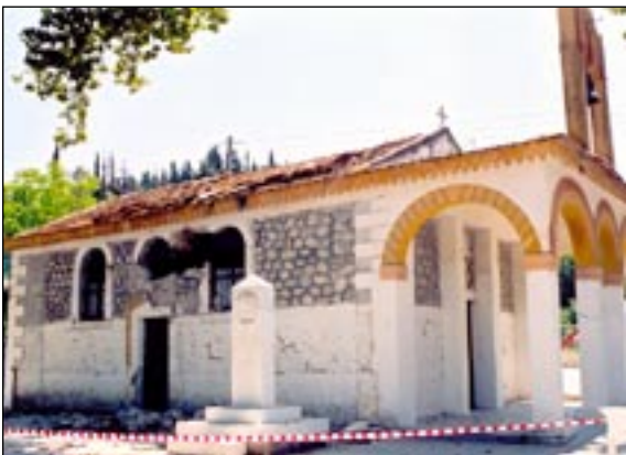
Figure 23. Cracking of masonry walls of Agios Minas church (town of Lefkada) (ITSACK team).
