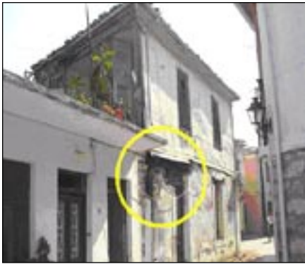
Figure 18. Partial collapse of masonry wall in a category B building (ITSAK team).
