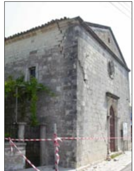
Figure 22. Churches built of stone masonry suffered heavy damage. In various parts of Lefkada, the tiles at the center of roofs moved. This might be explained by the vertical flexibility of the roof at its center (NTUA-UoA team).
