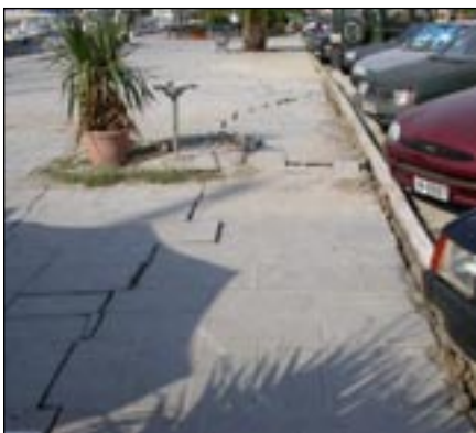
Figure 11. In the town of Lefkada, distorted pavement and sidewalks due to ground settlement and lateral spread (ITSAK team).
