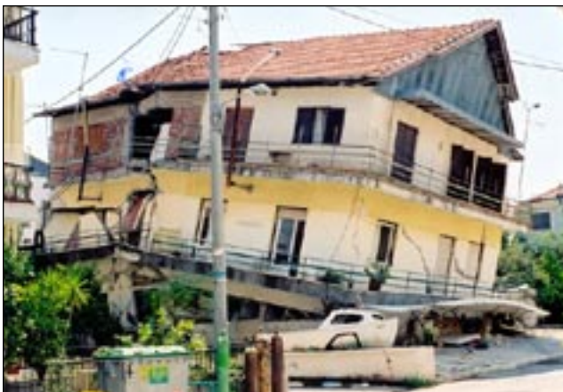
Figure 19. Collapse of R/C building in the town of Lefkada. On the right side, there are no brickwalls on the ground floor, where the building collapsed. The remaining part on the left side has partitions down to the foundation (NTUA-UoA team).
