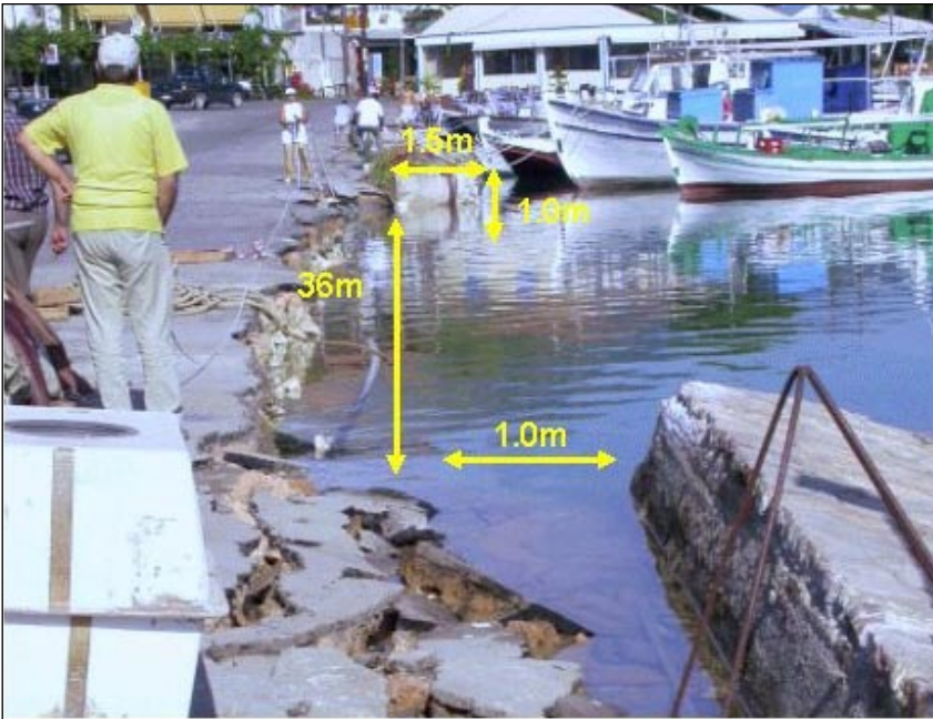
Figure 13. Part of the seawall has been laterally shifted and overturned (ITSAK team).
