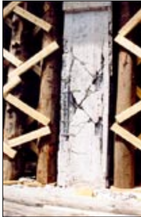
Figures 21a and b. A four-story building with a mezzanine was heavily damaged in the ground floor columns. The columns seem to have swollen in the center due to insufficient transverse reinforcement (NTUA-UoA team).
