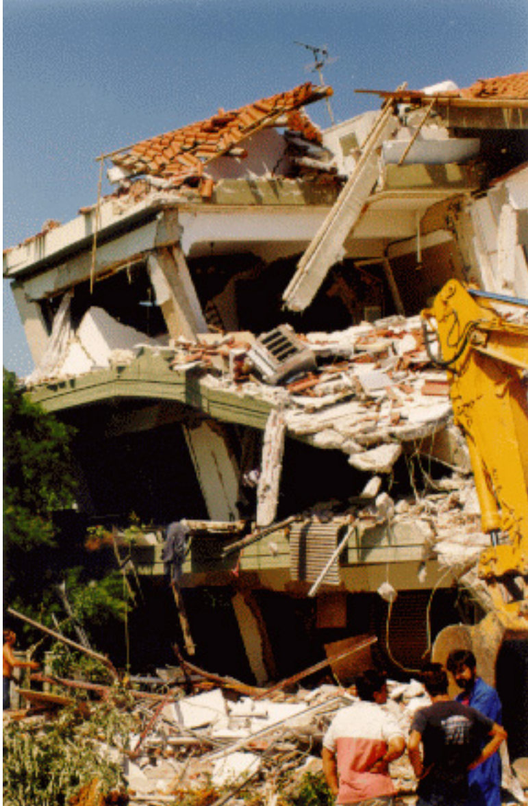
FIGURE 5B: Building Collapse in the 1999 Athens earthquake
