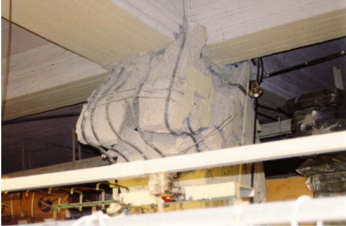
FIGURE 5D: Typical Earthquake Damage-Column Failure (1999 Athens Earthquake)
