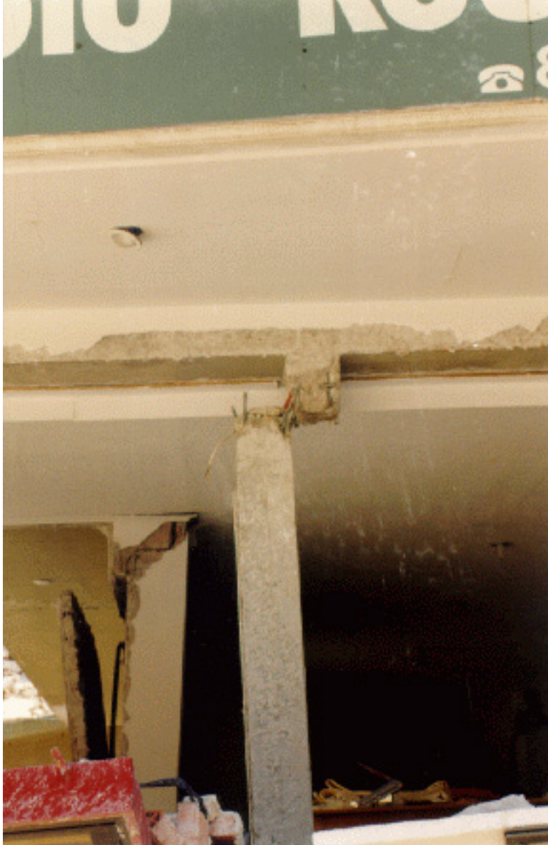
FIGURE 5C: Earthquake Damage- Dislodged Column due to Soft Ground Floor Effect (1999 Athens earthquake)
