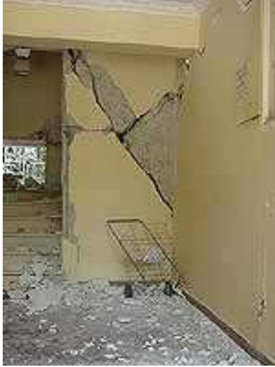
FIGURE 5F: Typical damage to the shear wall surrounding the stairwell in an apartment block in the 1999 Athens earthquake (Source: EQE)
