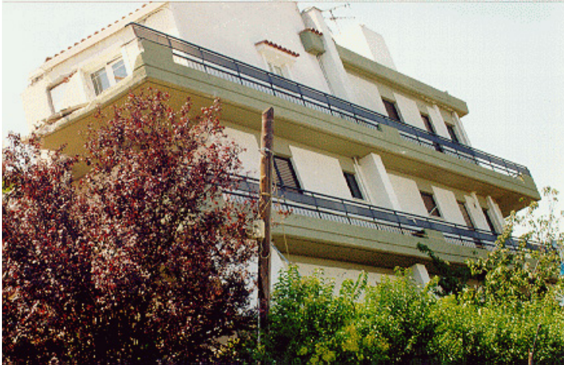
FIGURE 5A: Typical Earthquake Damage (1999 Athens earthquake)
