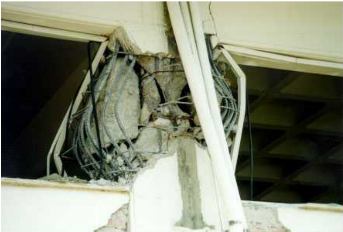
FIGURE 5E: Failure of column, due to short column effect, of a 5-storey building in Ano Liosia, which was built in 1997 according to the new Greek Seismic Code (1999 Athens earthquake); Source: ITSAK
