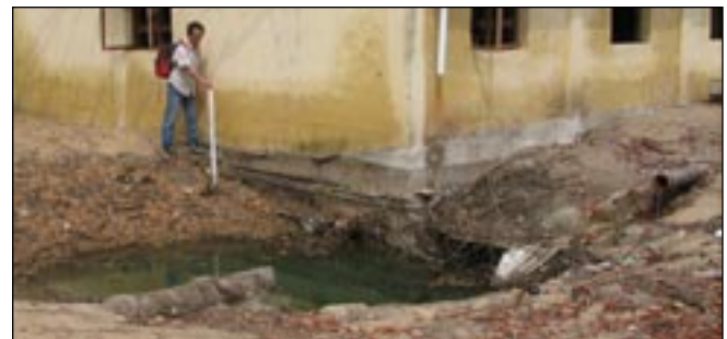
Figure 5. Tsunami scour and failure of a wastewater pipe at a schoolhouse at Kalapakkom.
