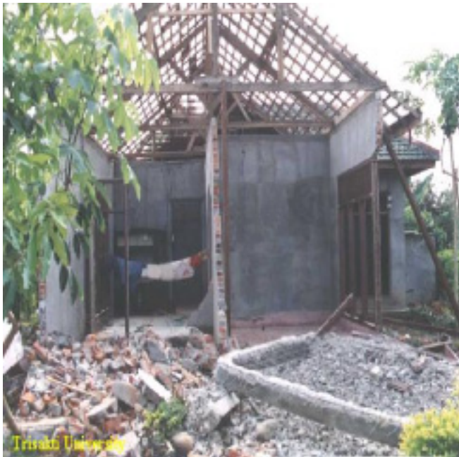
FIGURE 6A: A Photograph Illustrating Typical Earthquake Damage (June 4, 2000 Bengkulu Earthquake)
