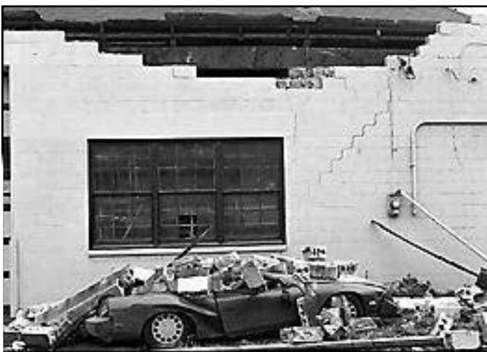
Collapse of a Seattle URM building in the Nisqually Earthquake.
