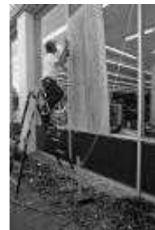
Broken windows in Napa, California following a 5.2-magnitude earthquake (AP Photo/Ben Margot)
