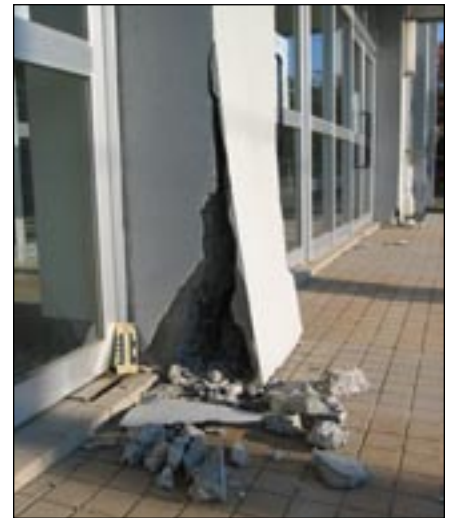
Figure 7. Damage to Urakawa Elementary School.
