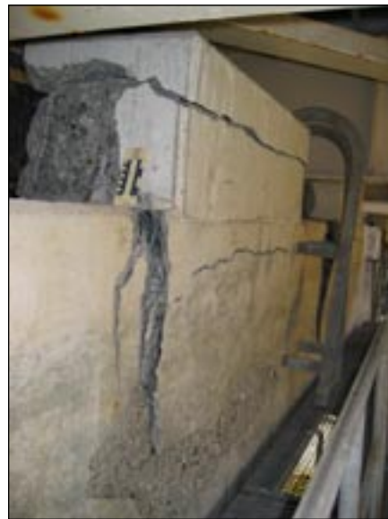
Figure 6. Damaged shear key from the Shizukawa Bridge near Tomakomai City.
