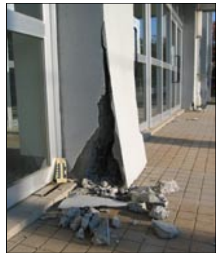
Figure 7. Damage to Urakawa Elementary School.
