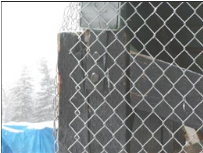
Figure 17 - Tetlin community building foundation damage
