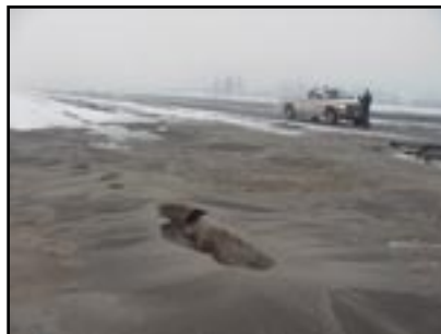
Figure 15 - Sandboils in apron
