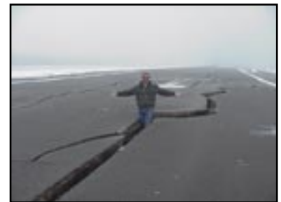
Figure 16 - Cracks in runway
