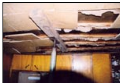
Figure 20 - Mentasta interior damage
