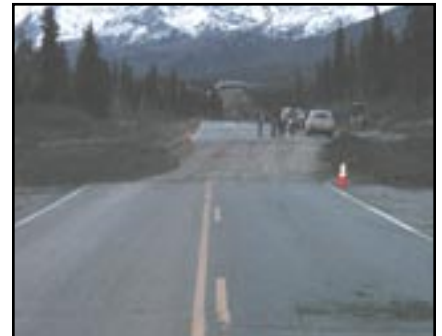
Figure 12 - Fault offset on Richardson Highway
