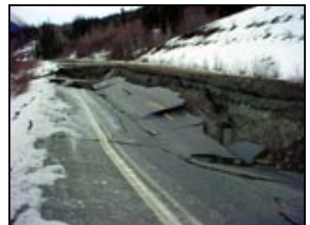
Figure 13 - Liquefaction-induced lateral spreading on Tok Cutoff
