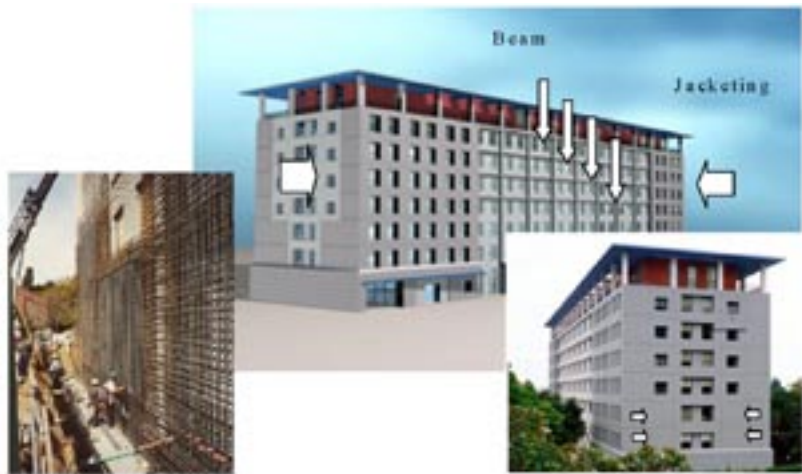
Barrows Hall at UC Berkeley, originally completed in 1964, was retrofitted in 2002 by Degenkolb Engineers. The jacketing scheme increased the strength and stiffness of the building by adding shear walls at the ends and allowed the building to remain inhabited during the construction process.
