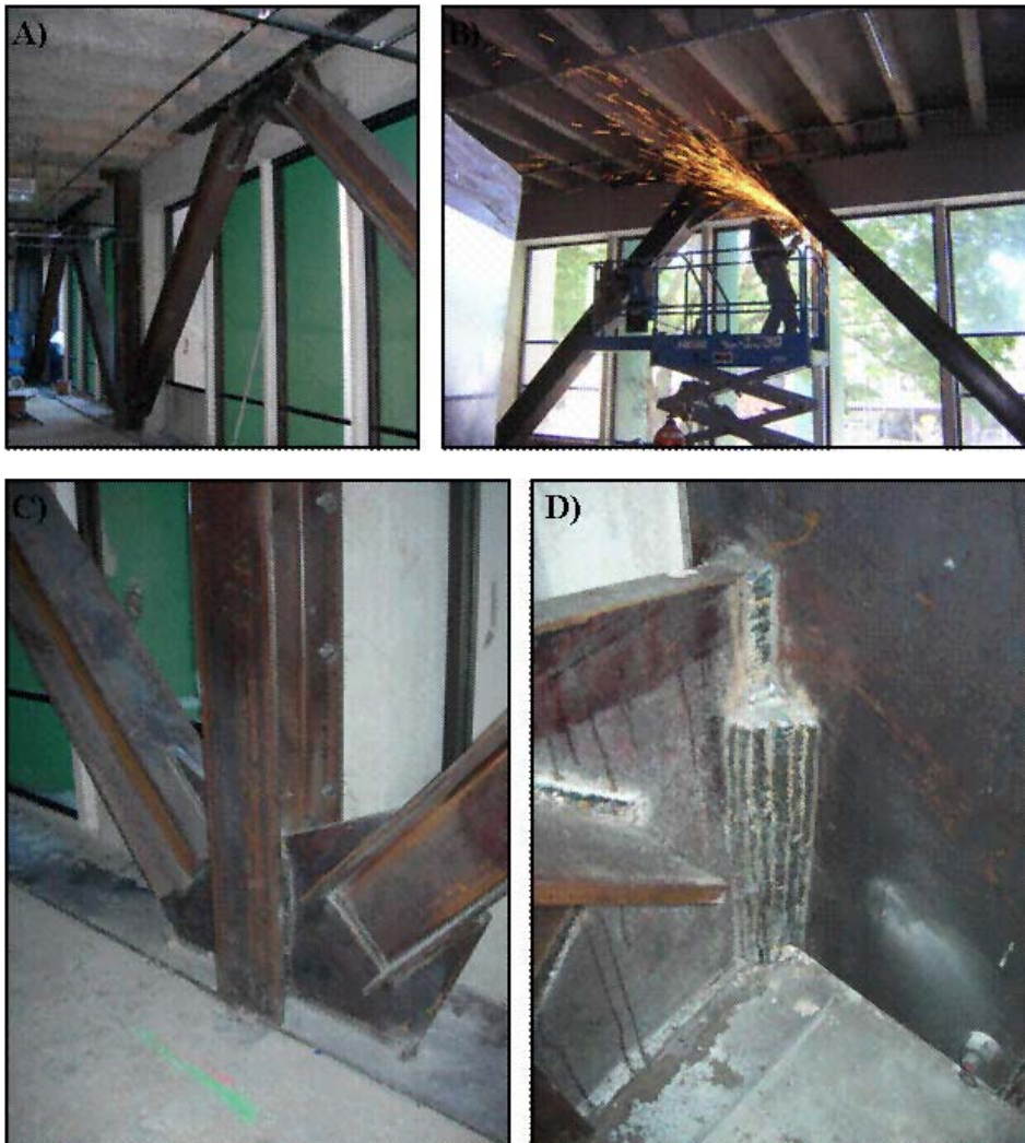
Construction of cross bracing on the first and second stories along the west elevation. (A) Installed cross bracing. (B) Cross bracing installation in progress. (C) Close-up of welded plate at floor level. (D) Close-up of weld used to connect new cross bracing to steel plates.
