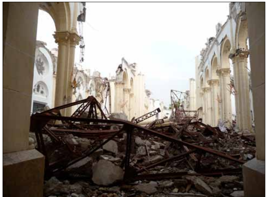
Figure 6. Collapsed roof, interior of National Cathedral, Port-au-Prince (photo: Martin Hammer).
