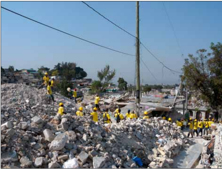
Figure 24. Cash-for-work for clearing debris from neighborhood school in the Nerette neighborhood of Petionville (photo: Rebekah Green).
