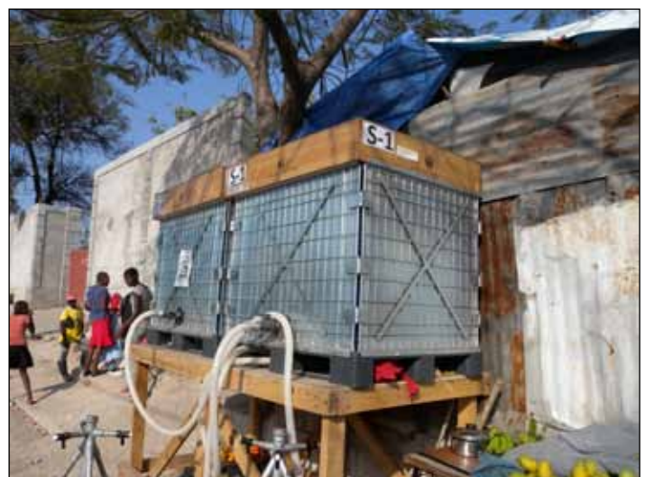
Figure 17. Emergency water tank (photo: Rebekah Green).
