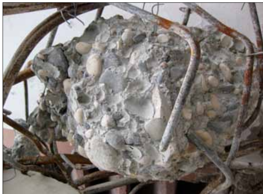
Figure 13. Lack of sufficient cement bond, smooth reinforcement, and insufficient detailing (photo: Anna Lang).
