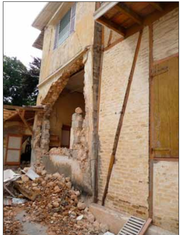
Figure 4. Colombage performed well, though the unreinforced masonry wall collapsed (photo: Martin Hammer).
