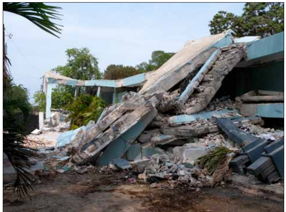
Figure 22. Damaged school in Port-au-Prince (photo: Rebekah Green).
