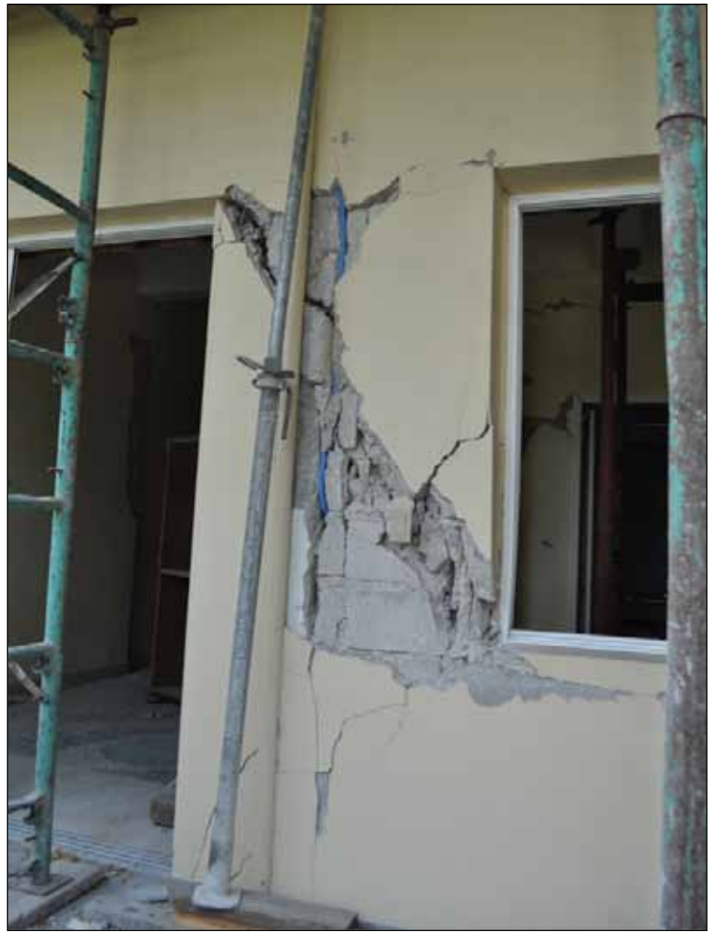
Figure 9 (left). Damage in a column due to captive condition, Petionville hotel (photo: Ayhan Irfanoglu).
