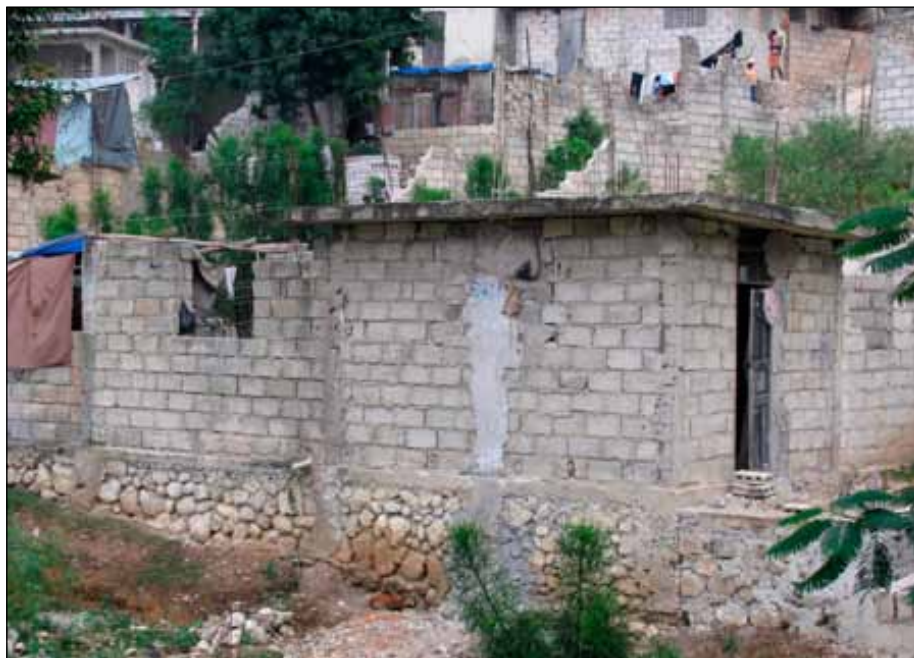
Figure 12. Typical construction of a residence, showing a rock rubble foundation, confined masonry construction technique, and reinforced concrete slab. Note blocks added to the top of the walls and reinforcement emerging from the slab, ready for construction of another level (photo: Anna Lang).
