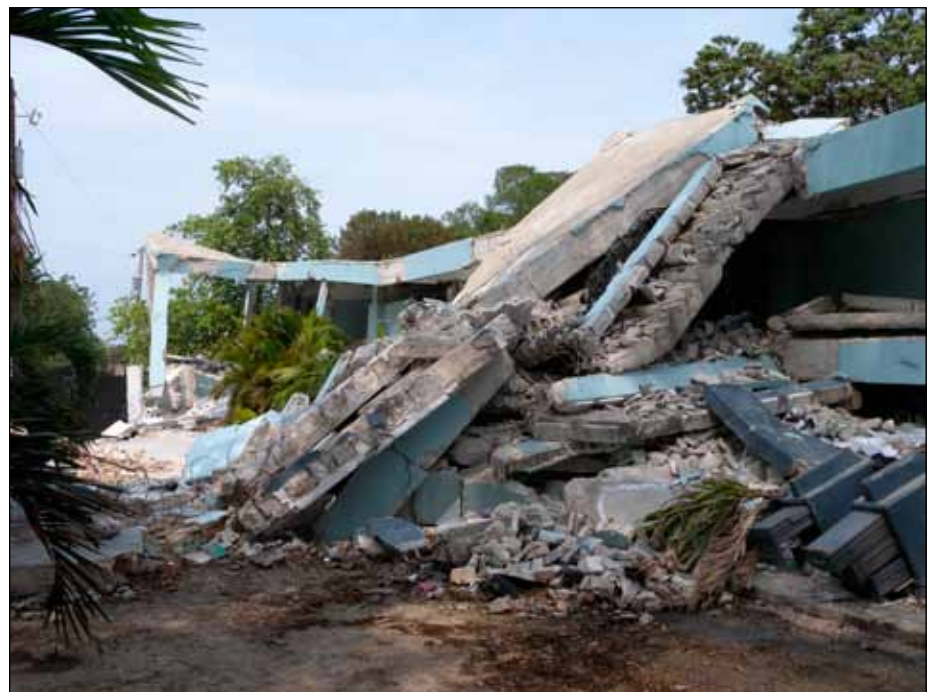
Figure 22. Damaged school in Port-au-Prince (photo: Rebekah Green).
