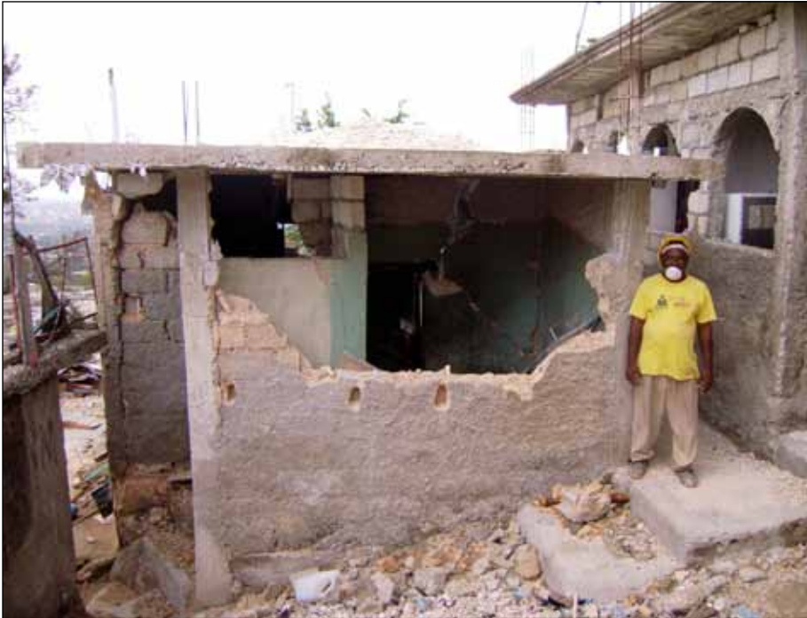
Figure 14. Typical out-of-plane failure of an infill masonry construction (photo: Anna Lang).
