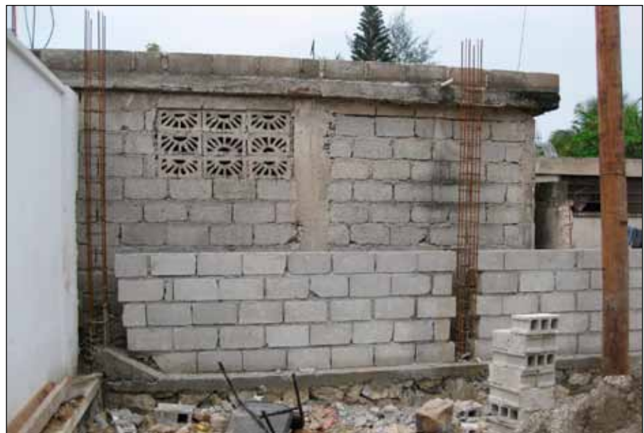
Figure 15. In foreground, new wall under construction shows staggering of blocks within the column cavity; this mechanically locks the masonry wall to the columns, causing them to act as a unit. In background, a typical one-story CM residence (photo: Anna Lang).
