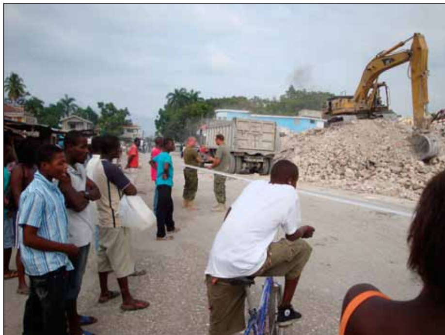
Figure 26. Canadian forces clearing debris of church in the town square of Léogâne (photo: Rob Olshansky).
