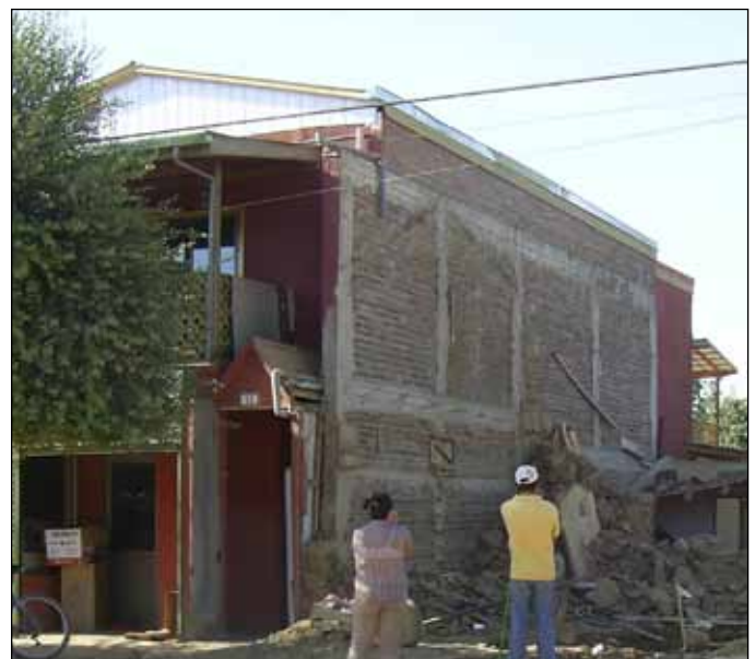
Good behavior of confined masonry building during the 2010 Chile earthquake (photo: Ofelia Moroni).
