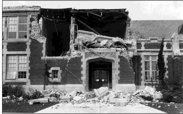
Fig. 7 – View of John Muir School, showing damage from the March 10, 1933 Long Beach earthquake. Located on Pacific Ave. in Long Beach, California. Photo taken on March 18, 1933 (photo: W.L. Huber) [15].
