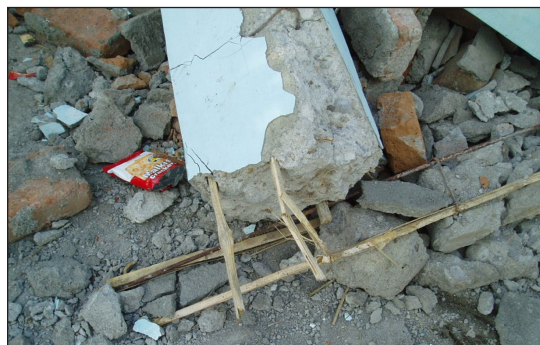
Poor joint detailing on collapsed building (photo: Teddy Boen).
