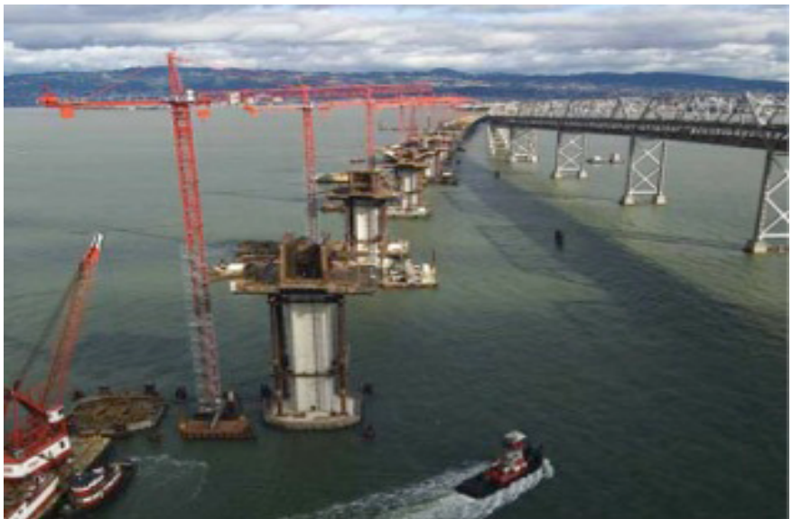
Construction of the replacement of the seismically-vulnerable San Francisco-Oakland Bay Bridge (source: CalTrans, 2002).
