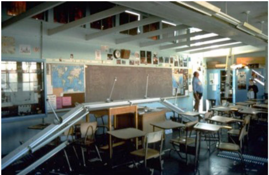
Lights fell onto desks in a Northridge Junior High classroom during the 1994 earthquake. School was not in session, so no injuries occurred. (photo: Gary L. McGavin, source: Reitherman et al., 1995).
