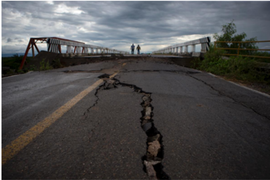
Bridge connecting Juchitan to Union Hidalgo in Oaxaca state, Mexico. Bridge survived but, the road leading up to each side fissured and the supporting walls buckled. (AP Photo/Rebecca Blackwell)
