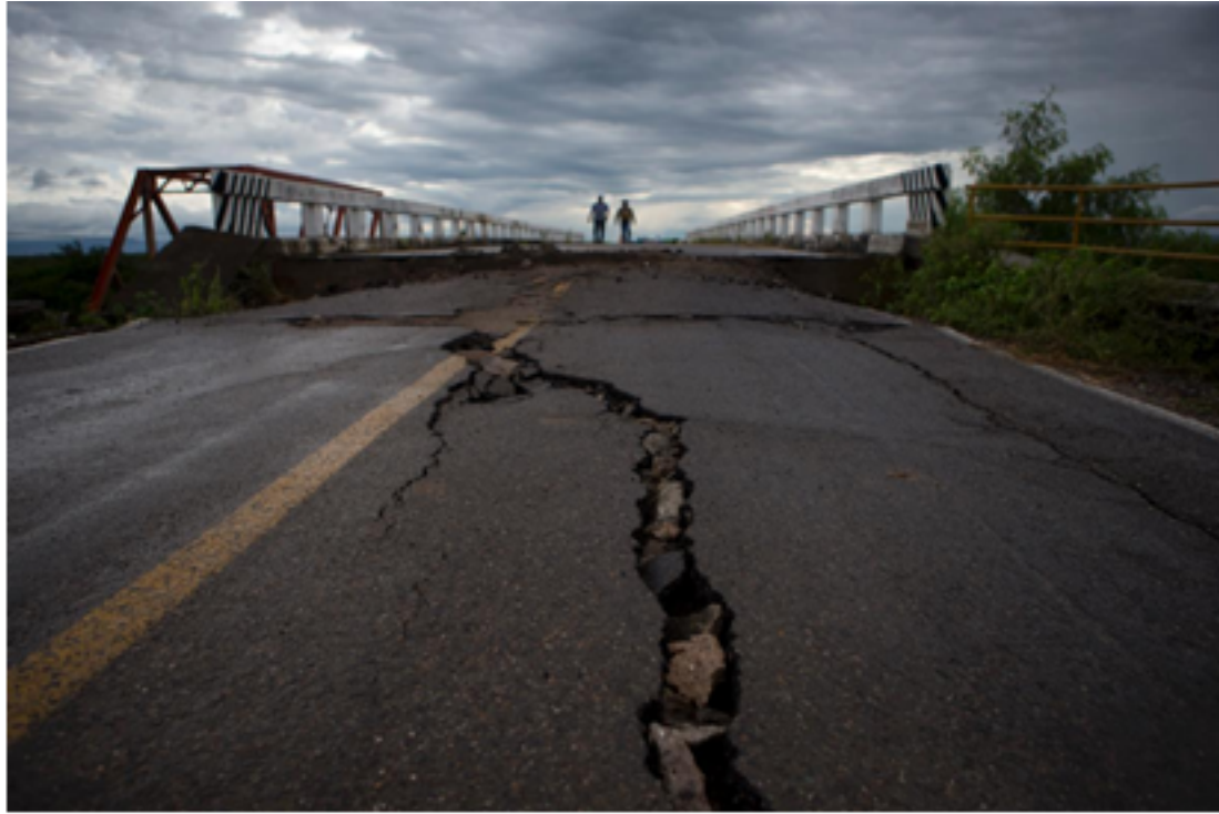
Bridge connecting Juchitan to Union Hidalgo in Oaxaca state, Mexico. Bridge survived but, the road leading up to each side fissured and the supporting walls buckled. (AP Photo/Rebecca Blackwell)
