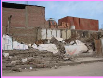
confined masonry in back , collapsed adobe in front
